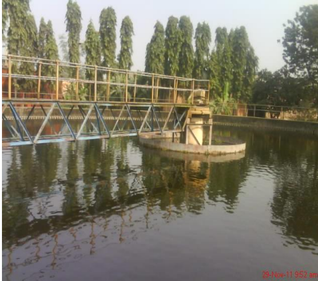
Picture 20: STP at Howrah
